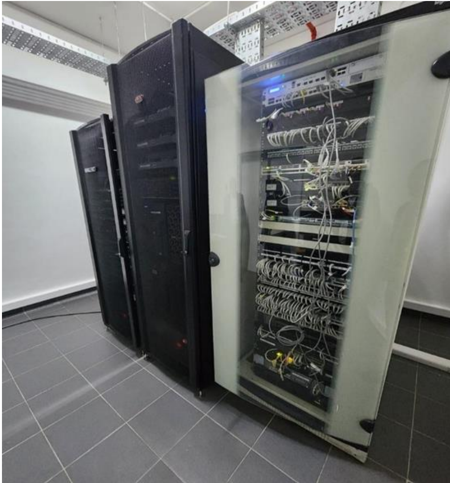
Server room at INAM
