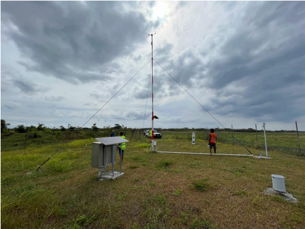
Figure 8 - Whitegrass International Airport – Automatic Weather Station
