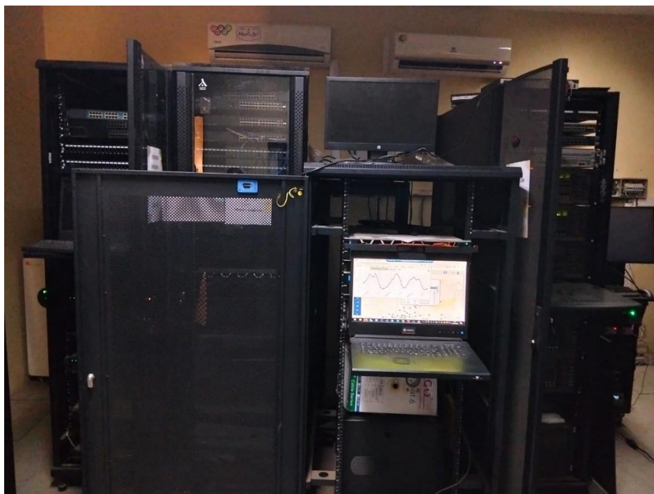
Figure 4: DNM Server Room in Niamey
